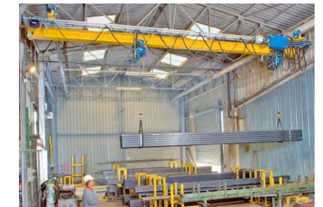
Single girder bridge crane
