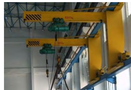
Wall traveling jib crane
