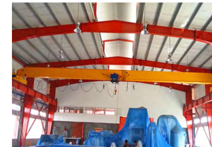
Single girder bridge crane
